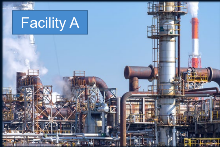
Oil combustion facility
